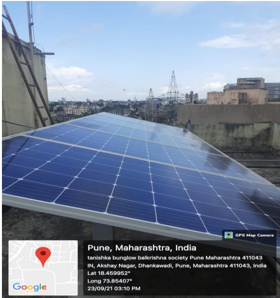
Solar Panel left Corner
