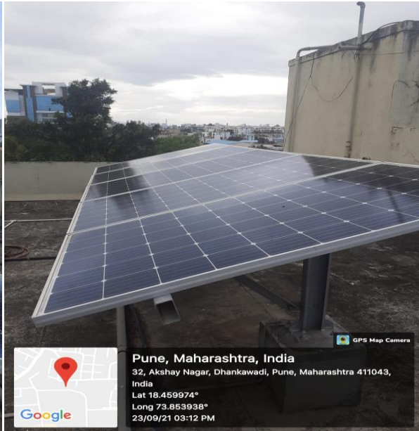
Solar Panel Right Corner
