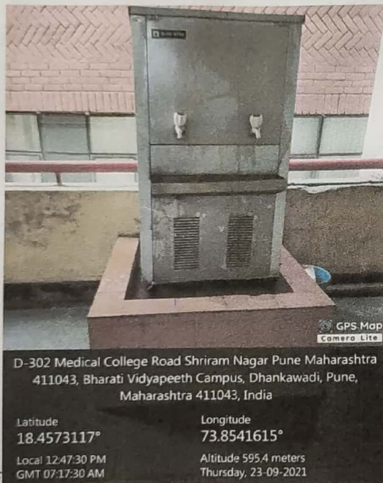
Figure 16: WATER PURIFIER SYSTEM
